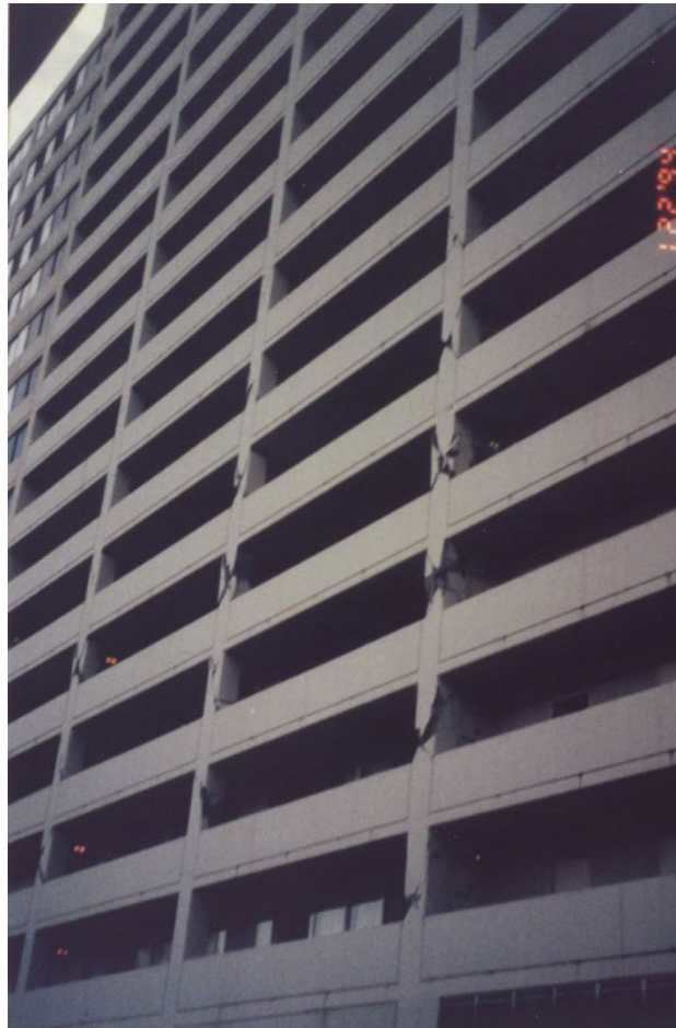
Damage from the 1994 Northridge earthquake to the perimeter moment frames of the Champaign Tower in Santa Monica, CA. [5]
