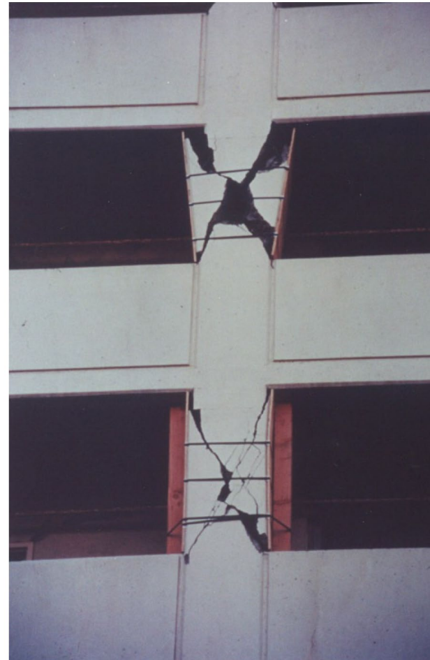
Balcony parapets induced short-column effects in the Champaign Tower moment frames. Typical X-shaped shear cracking from the short-column behavior is shown. [5]
